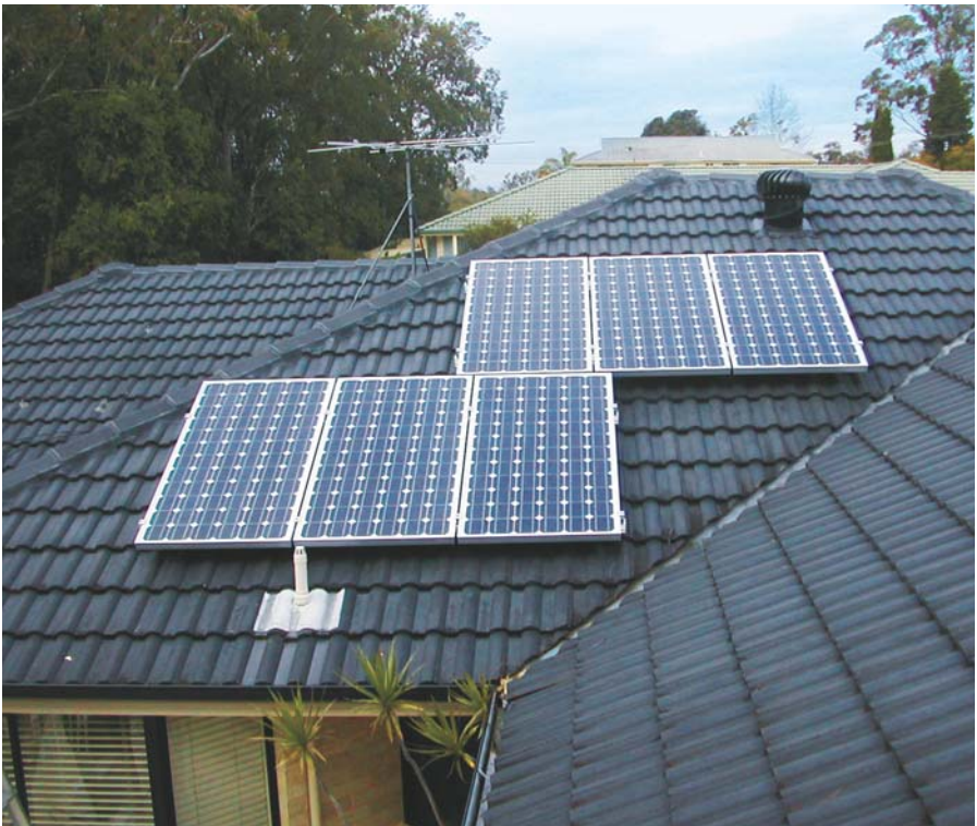
An example of a 1kW solar power system
